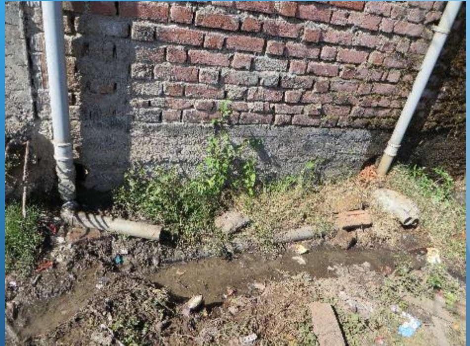
Unconnected Pipe releasing human waste
